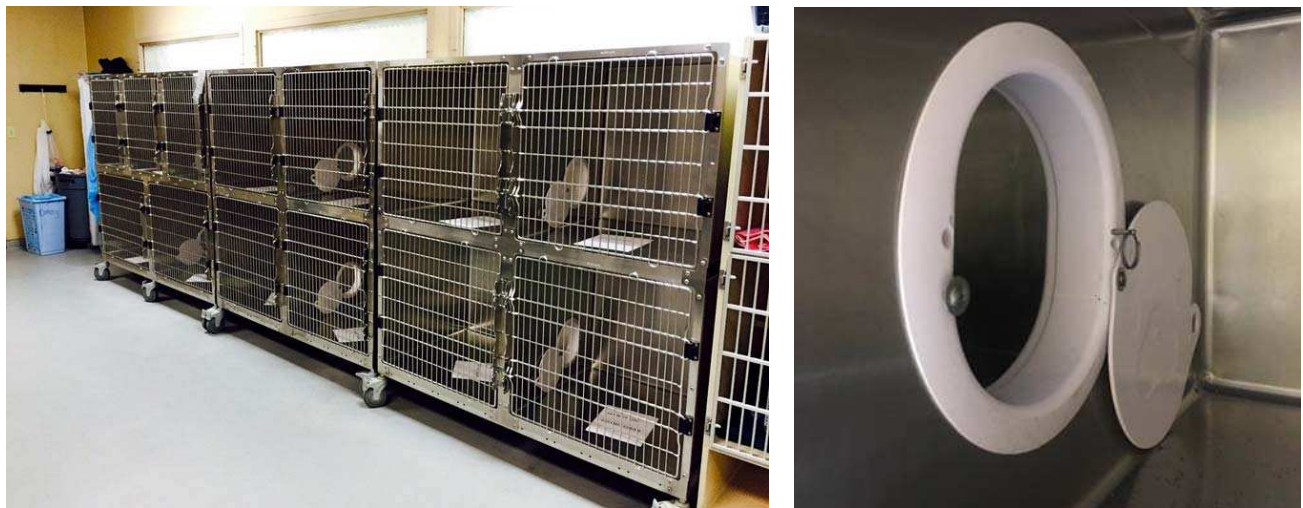
Figure 18: Shows an example of stainless steel cages retrofitted with one porthole between two cages. http://www.sheltermedicine.com/library/manufactured-portals-order-information-and-instruction-for-installation
