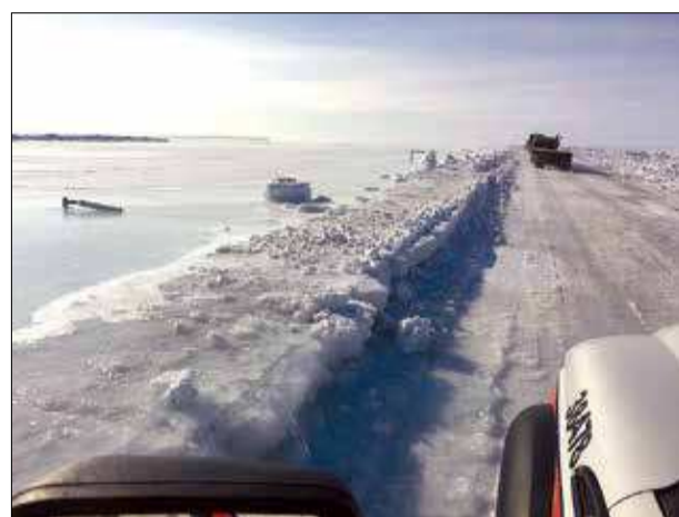
Overflow flooding is seen at approximately 400 Mile Dalton Highway. After briefly opening to traffic following initial overflow flooding, the highway has closed again. COURTESY ALASKA DEPARTMENT OF TRANSPORTATION
