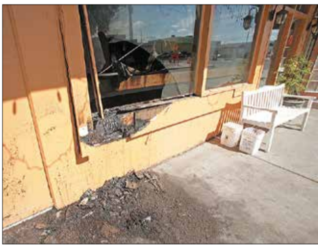
A fire caused damage at Gambardella's, seen here Thursday afternoon. ERIC ENGMAN/NEWS-MINER
