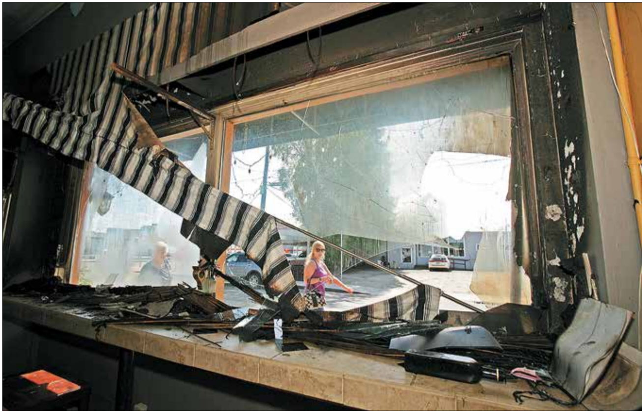
A fire started by a cigarette butt in a flower planter box outside Gambardella's restaurant damaged the front of the building, seen from inside the restaurant Thursday afternoon. ERIC ENGMAN/NEWS-MINER
